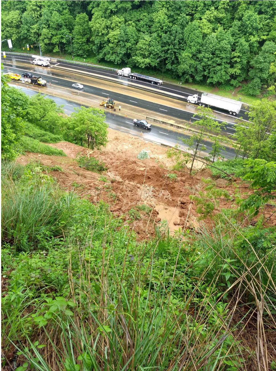
May 30, 2018. Top of current scarp. Slide blocked WB lanes and jumped barrier to EB lanes.
