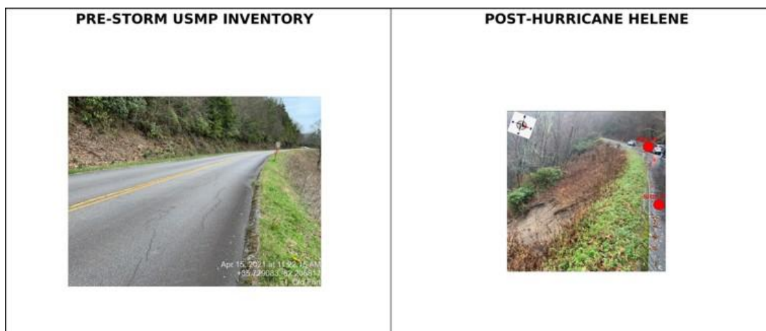
Figure 6. Pre- and Post-Storm Conditions at MP 348.9. Left: pre-storm USMP view at MP 348.8. Right: post-storm slope failure and boring locations BH25-15 and BH25-16.
