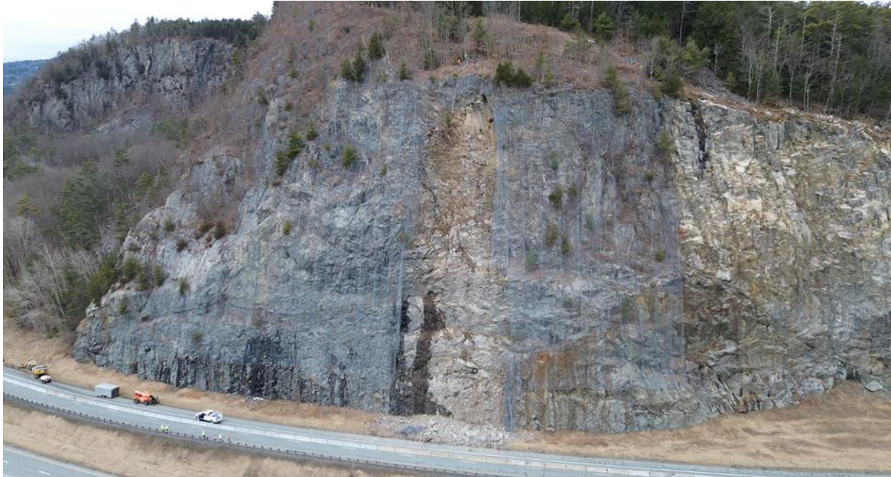
Figure 4 – Drone image of scalers beginning emergency response on March 5, 2024, following the February 27, 2024 rock fall (VTrans)
