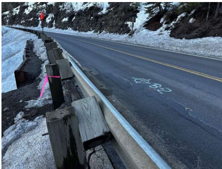
Figure 2 – NB Lane Showing Cracking Prior to Failure, Photo Taken March 3, 2025
