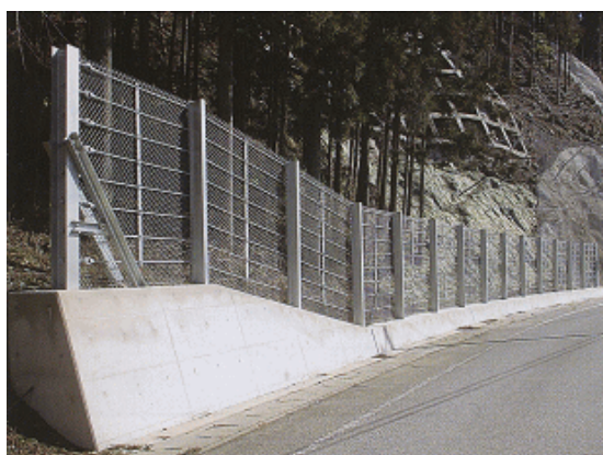
Figure 1 - Standard-Type Rockfall barrier
