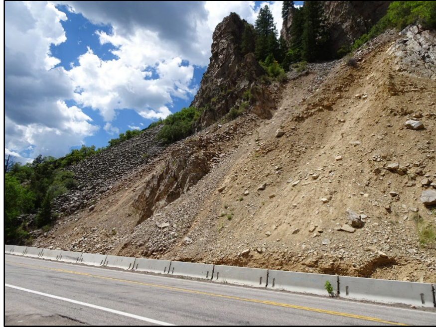
Figure 10 – CO 133 slope cut into talus slope forming a long term erosional and maintenance issue.
