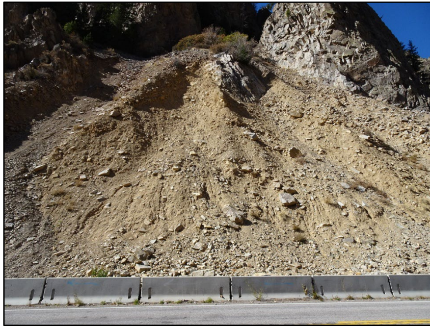
Figure 9 – CO 133 slope cut into talus slope forming a long term erosional and maintenance issue.
