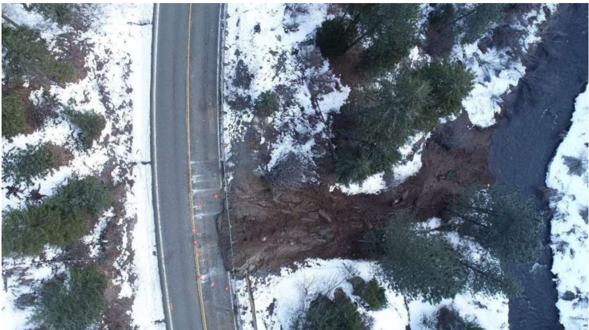
Figure 3 – Overhead View of Failure, Taken with Drone on March 19, 2025
