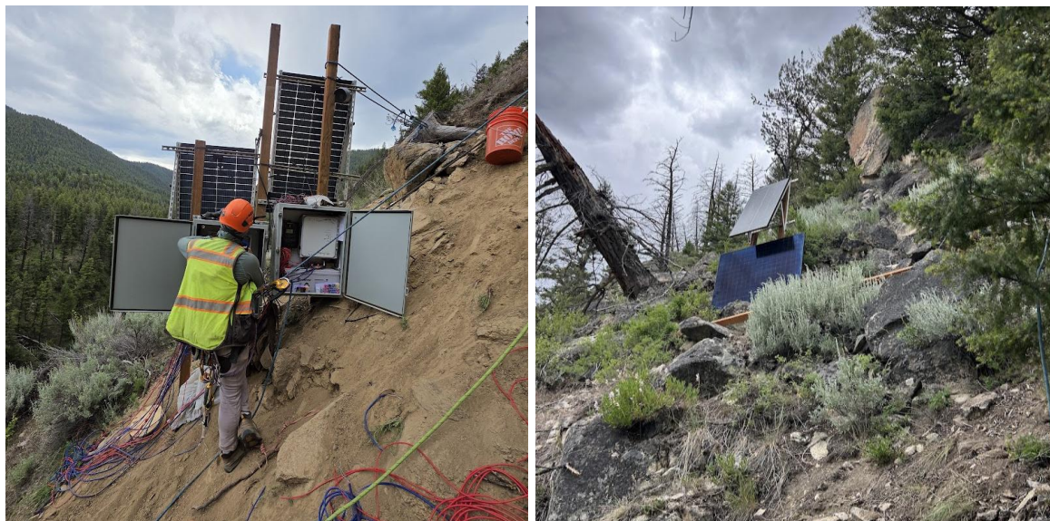
Figure 11 – Wiring on System 10_11 (left) and Solar Array on 5_6 (right)
