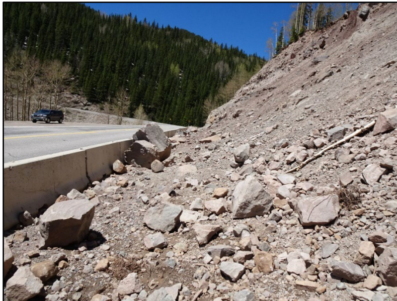
Figure 14 –US 550 Deer Creek. Side view of slope that was cut to accommodate roadway leaving an over steepened erosional rockfall prone slope.
