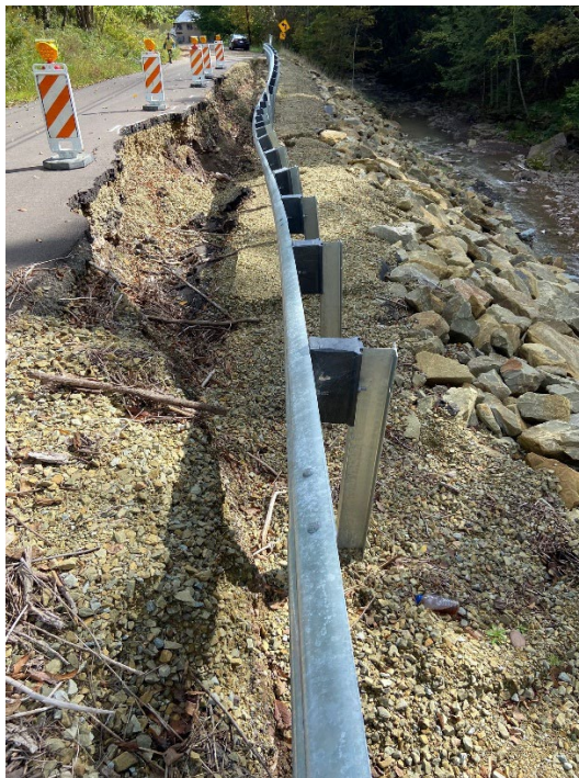
Photo 5: Failure of Repairs at Site 1
