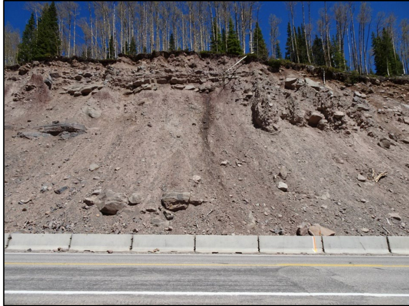
Figure 13 –US 550 Deer Creek. Slope that was cut to accommodate roadway leaving an over steepened erosional rockfall prone slope.
