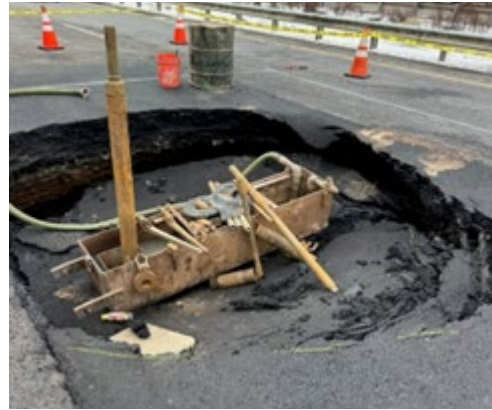
Photo of Mine Subsidence Location 2
