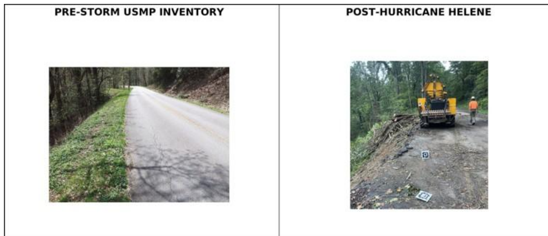
Figure 4. Pre- and Post-Storm Conditions at MP 345.7. Left: pre-storm USMP view. Right: post-storm roadway-edge failure and debris.
