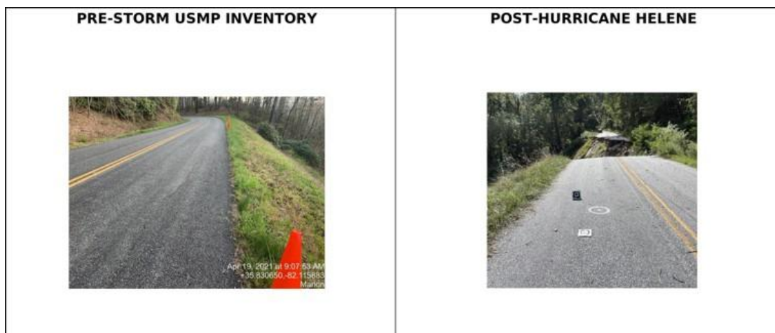
Figure 2. Pre- and Post-Storm Conditions at MP 336.7. Left: pre-storm USMP photograph at MP 336.6. Right: post-Hurricane Helene roadway washout at MP 336.7.
