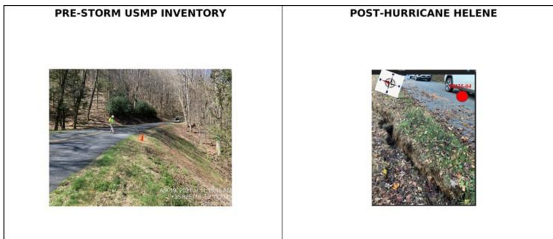
Figure 3. Pre- and Post-Storm Conditions at MP 338.2. Left: pre-storm pavement cracking. Right: post-storm outside-shoulder deformation near MP 338.2.
