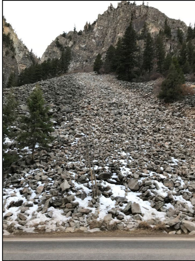
Figure 1 – Existing Talus Slope in Colorado. Left (darker colored) side is non-displaced talus. Right (lighter colored) side is an example where the toe was disturbed and triggered the entire slope to move downhill to re-establish the existing angle of repose.
