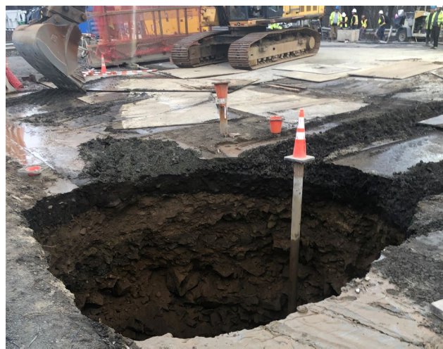
Photo of Mine Subsidence Location 3
