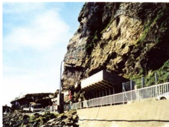
(b) After the rockfall
