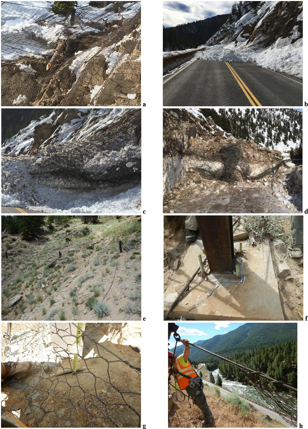
Figure 5 – Photographs of Typical Avalanche Damage, February 15, 2017 (a, b, c, & d) and from Later Detailed Repair Design Reconnaissance (e, f, g, & h). All Photos from WFL.
