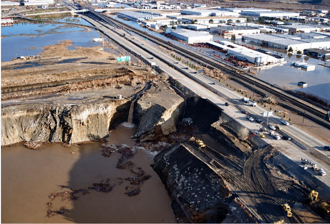
Figure 6. The January 1997 flood breach: floodwater from the Truckee River undercut and collapsed the wall of Helms Pit, eroding the shoulder of westbound I-80.
