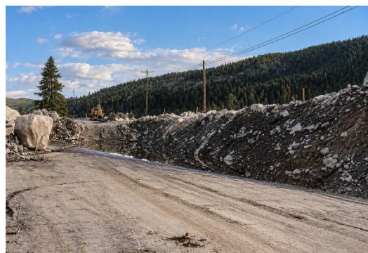
Figure 21. Bouldery slide deposits 6 ft thick being cleared from Bowers Mansion Rd. (RGJ).
