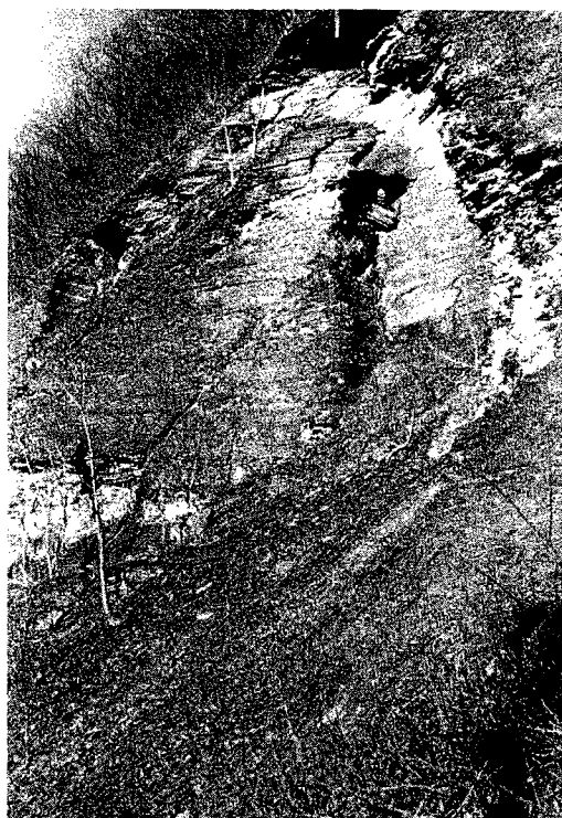
Figure 11: Plane failure at East Steubenville cut.
